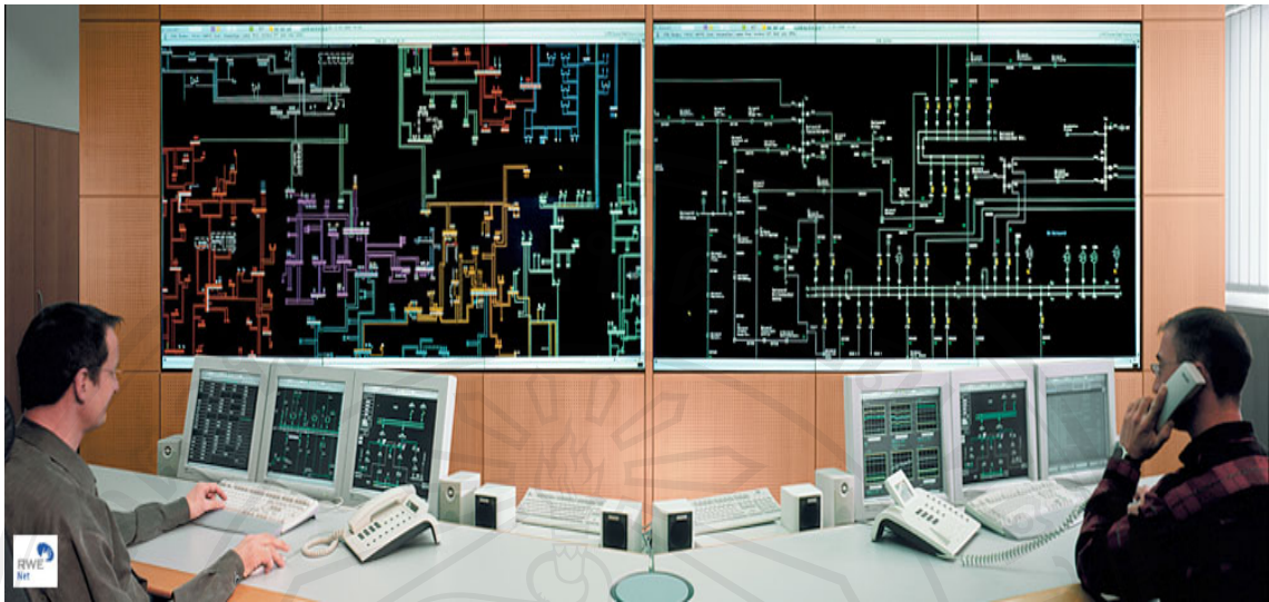
Figure 2.10: Operator Console and Wall Display
