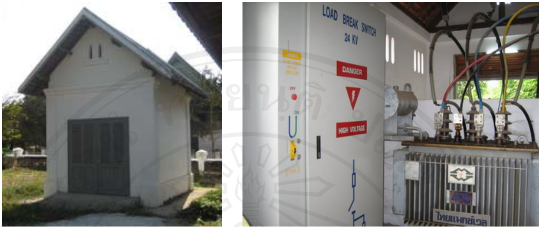
(a) substation house
