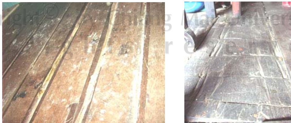
Fig.3.45 The poor-quality planks used as the substitutes for the original ones with the covering of sticking-plasters on opening slits in between (left).
