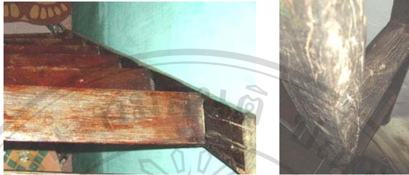
Fig.3.37 The cracks on the wood surface of the stairs caused by thermal movement.
