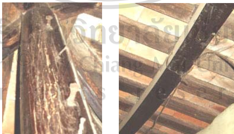
Fig.3.56 Iron nails fixed on timber elements cause rots of them.
