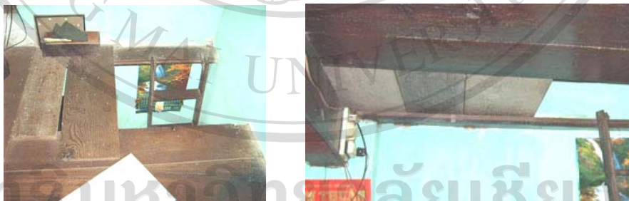
Fig.3.41 The encroachment of the stair-holes by disordered wooden planks has affected the outstanding characteristic of the timber stair.
