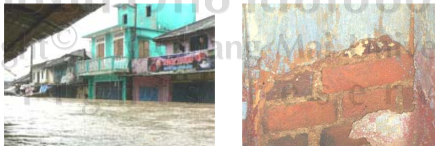
Fig.3.32 The flooding in Bao Vinh (in 2008) and the flakiness of the plaster and finishing on the below parts of the load bearing walls caused by flood.
