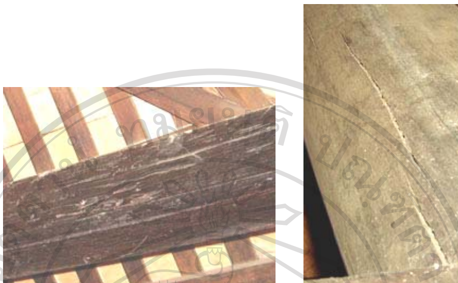
Fig.3.51 Cracks caused by thermal movement appear on the horizontal (left) and vertical trusses (right) of the timber frame system.
