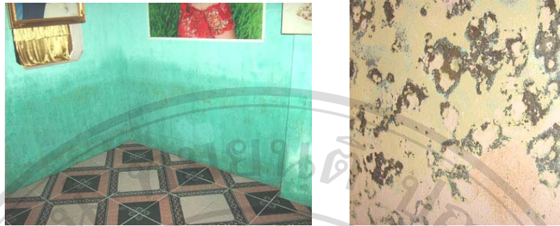
Fig.3.31 Fungi and moulds have grown on the below part of the walls on the ground floor (left side) and on the 2 nd floor (right side).
