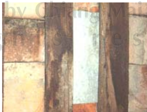
Fig.3.54 Iron plate is used to seal the holes on the roof for water-proof.
