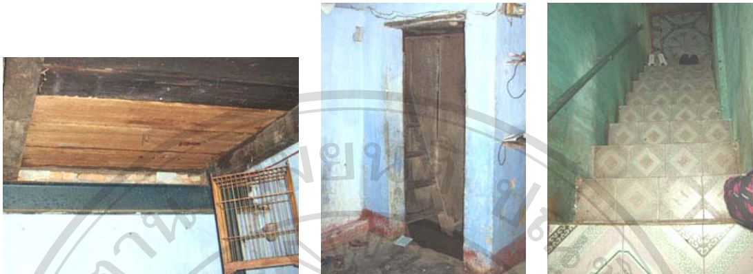
Fig.3.40 The moving to the other place outside the original structure of Tu Giac house and its stair hole left with the new wooden planks (2 photos on left sides). The changing into new material of concrete of the timber stair (right side).
