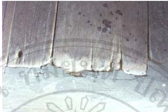
Fig.3.48 Deterioration of the endpoints of the timber floor planks.
