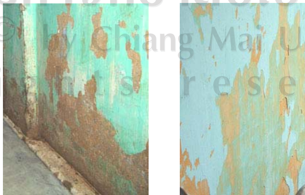
Fig.3.34 The flakiness of finishing layers, the calcium-originated whitewash, on the load bearing walls.
