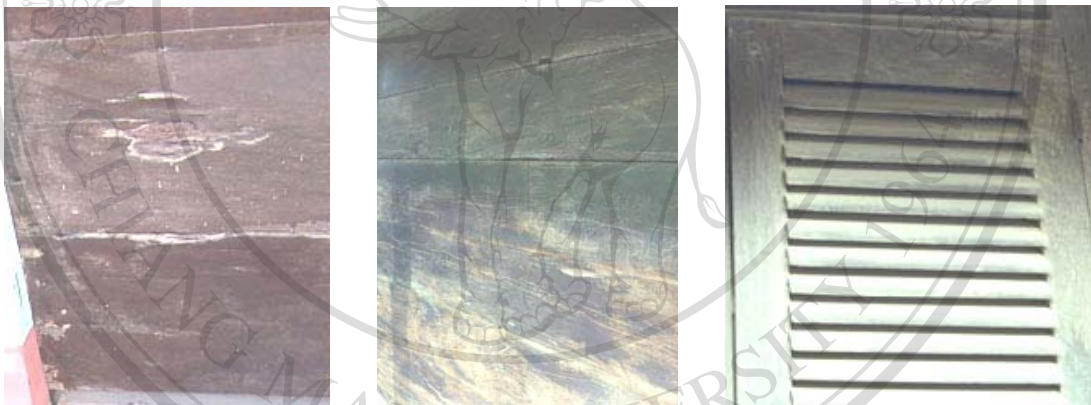
Fig.3.57 Holes, cracks and rottenness are created on the surfaces of wooden doors and windows by pest and fungal attacks and the aging process of wood.
