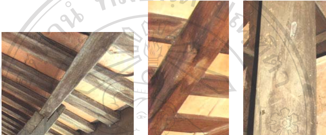
Fig.3.50 Fungal attacks (left and middle) and termite attacks (right) on the elements of the timber frame system of hip roof.
