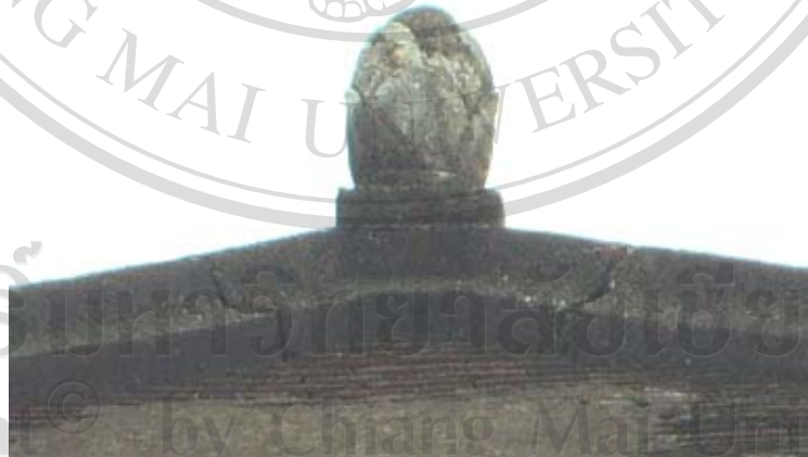
Fig.3.49 The cracks of the roof ridges on the top.
