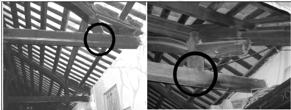
Figure 6-2: The condition of Tron Cot in HTGHs
