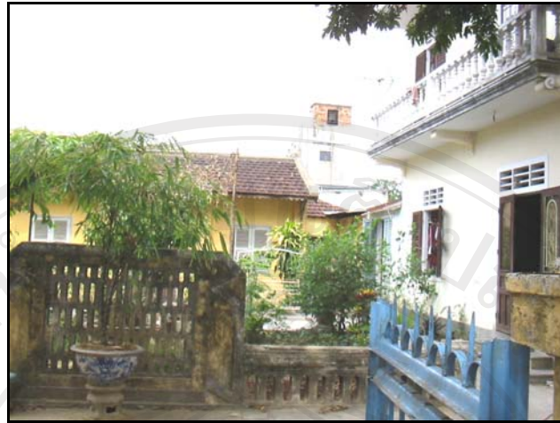
Figure 6-15: New two-storied structure for flood protection in HTGH B03 has broken the emphasis representative of Nha Chinh
